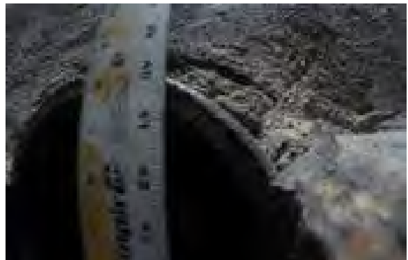
Monitored Pipe Size
