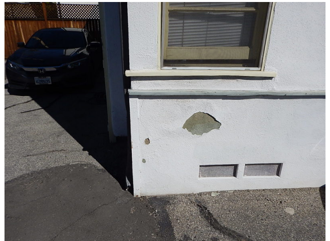
20. View of typical paint damage on exterior of subject property building
