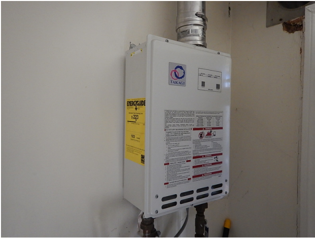
17. View of tankless water heater in laundry room at subject property
