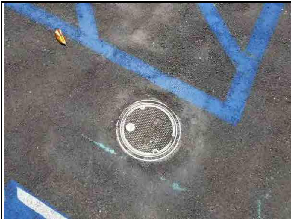
9. View of one of the five on-site groundwater monitoring wells.
