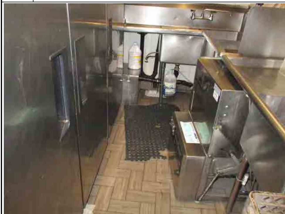
16. Floor-mounted grease trap at restaurant.
