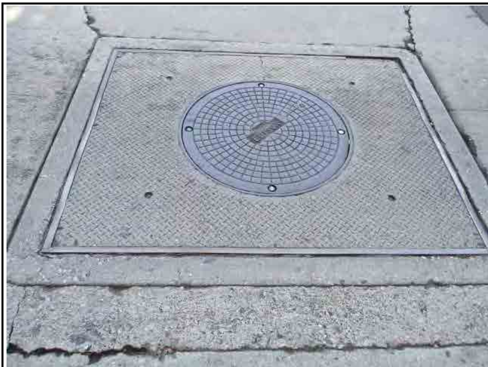
13. Offsite vault-mounted transformer located along public roadway.
