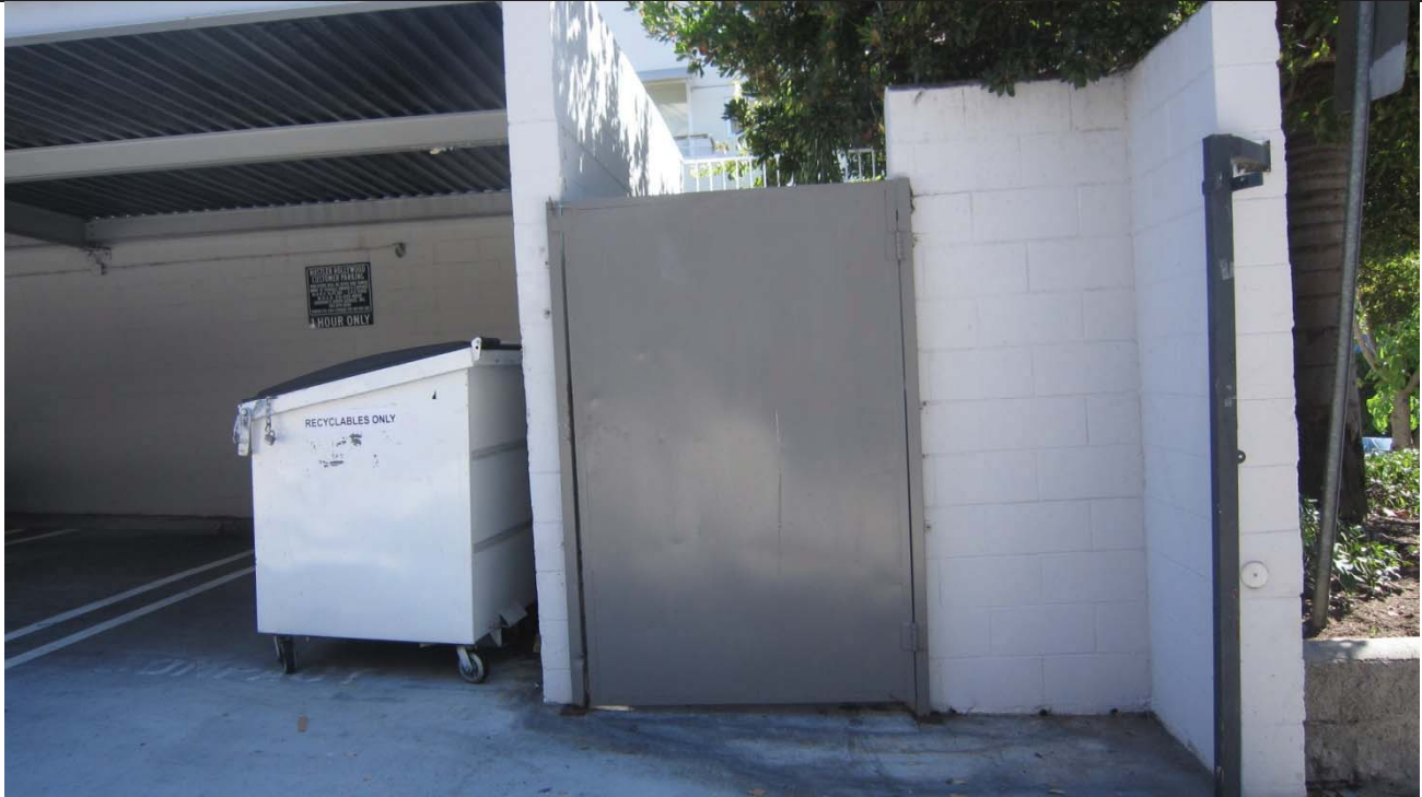
PHOTO 5: View of waste disposal area located in the southwest corner of the Site.
