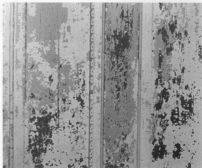
Figure 11. A dark layer can be seen beneath the flaking lighter paint on these raised field panels. Depending on the project work goal and the period of the building's history being interpreted, any one of the paint layers could be duplicated in repainting. National Park Service files.
