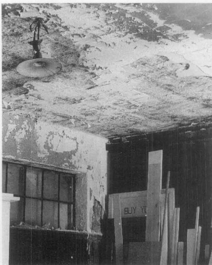
Figure 13. Part of a historic freight depot, this is not a high-style room and its painted surfaces are obviously in poor condition from long-term neglect. Interior spaces that are being converted for a new use in rehabilitation projects can benefit from being repainted in historic period colors rather than a neutral off-white. Photo: National Park Service files.
