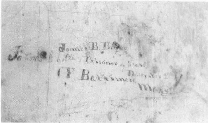
Figure 12. When discovered, important examples of history such as this pencilled Civil War graffiti should be preserved. A conservator can easily clean the area, then apply a protective coating. The history this hand-written message possesses is well worth the sacrifice of surface uniformity, even if it interrupts a freshly painted surface. Photo: Kaye Simonson.
