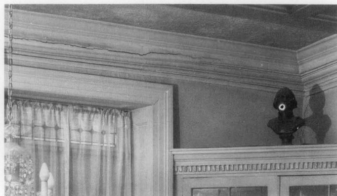
Figure 18. The major crack along this cornice indicates that there has been long-term moisture problem in this room. Restoring the plaster work and repainting should be done only after the water problem is solved. Photo: Jack E. Boucher for HABS.
