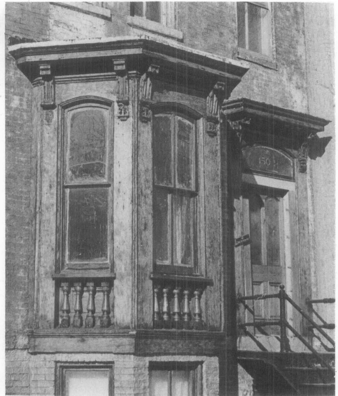
Fig. 2 A traditionally painted bay window has been stripped to bare wood, then varnished. In addition to being historically inaccurate, the varnish will break down faster as a result of the sun's ultraviolet rays than would primer and finish coats of paint. Photo: David W. Look, AIA.
