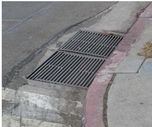
Figure 7.15 Improper Drainage Grate Design
